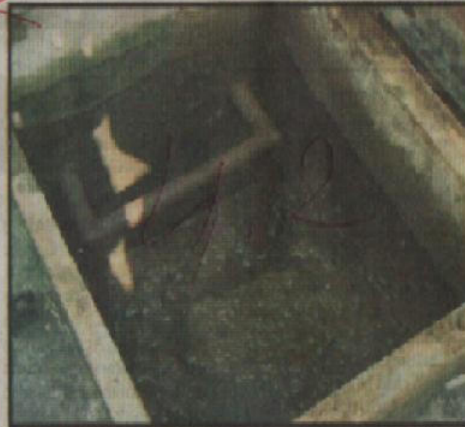
Sludge accumulated inside the reservoir of the PHE at Mawlai Motsyar which supplies drinking water to the people of Mawlai. (ST)
