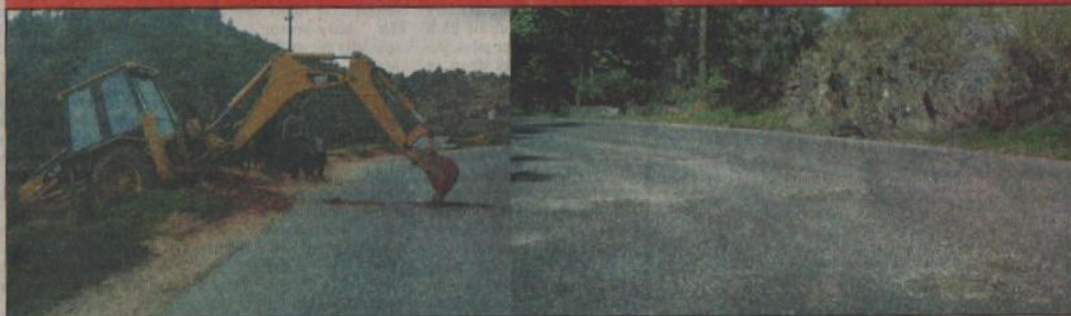
(L) A JCV which fell into a gorge is being lifted onto the road resulting in damage to the road which had been recently repaired. (R) The large holes visible on the Guwahati-Shillong highway which had been recently repaired by the State PWD. (Photos contributed)
