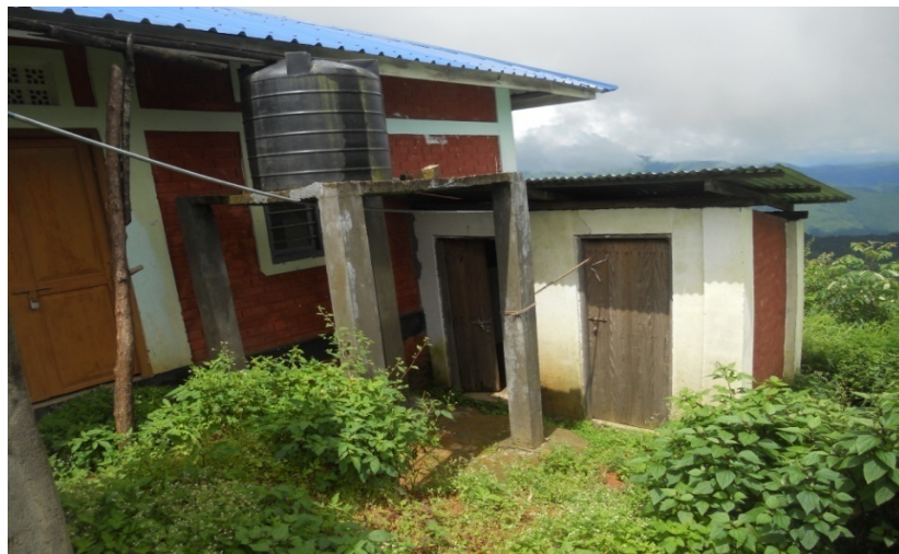
ii. Unused toilet of Phungyar PHC due to bad condition
